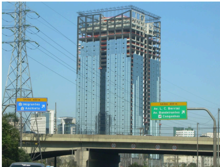
Figure 11 - OODC charged in building in São Paulo
