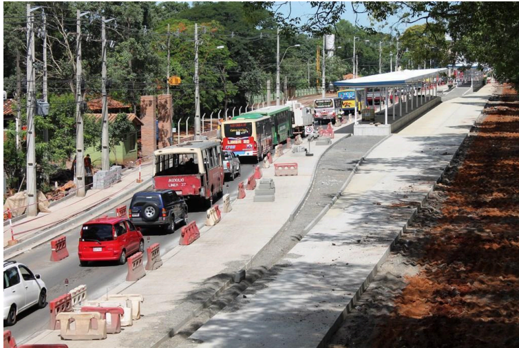
Figure 46 - Partially built BRT in Asuncion that has been destroyed as the project was aborted.
