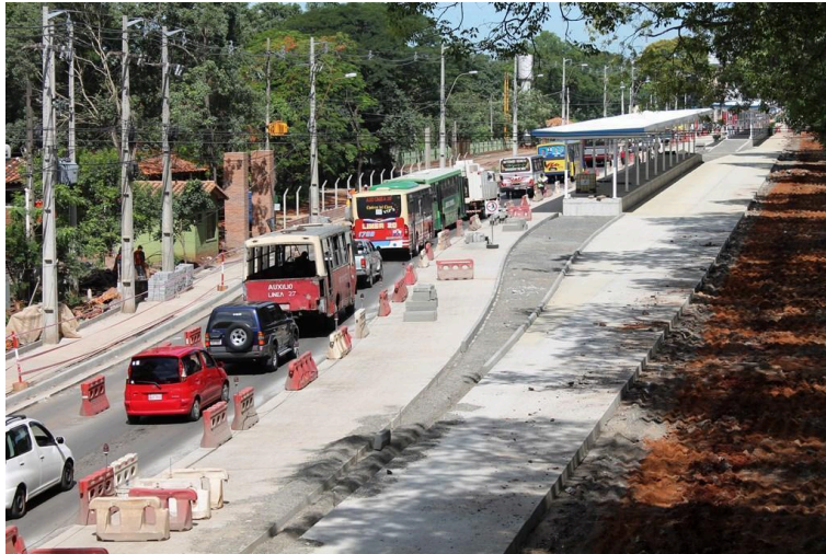
Figure 46 - Partially built BRT in Asuncion that has been destroyed as the project was aborted.
